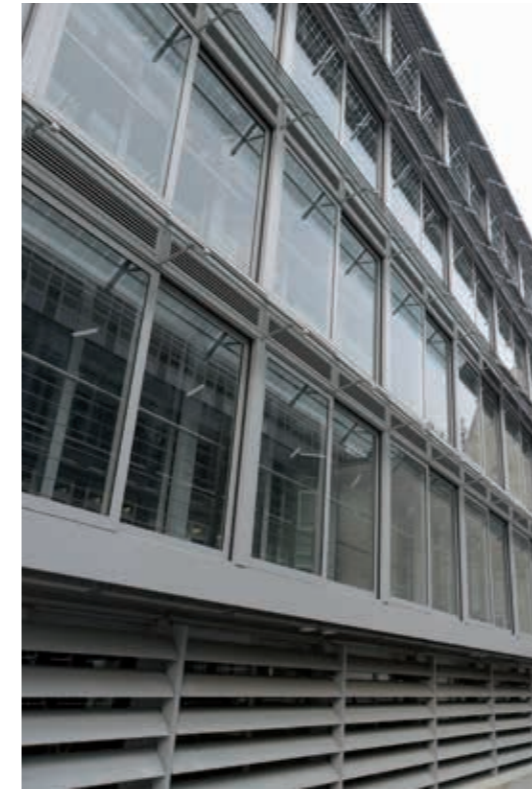
Fig 7 Photovoltaic solar shading
