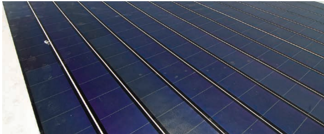
Fig 2 Thin film PV mounted on roof
